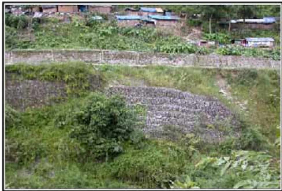
Plate 2.2 Ghate Khola landslide cone
