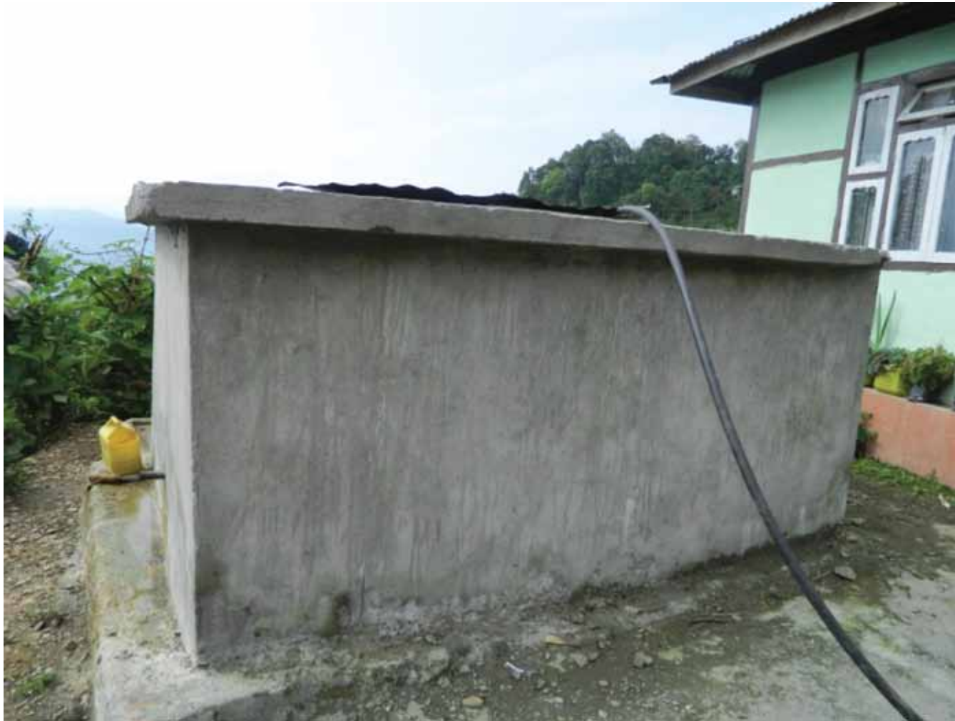
Water supply and storage: tanks made by RMDD for Rainwater Harvesting, in the non rainy season being used as storage tanks (the top of the tank is temporarily covered by a CGI sheet)
